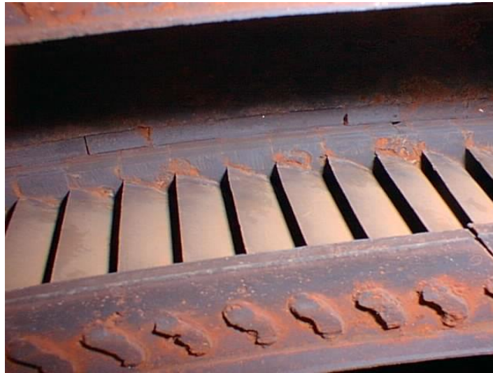
Figure 41 Turbine Blade Corrosion
